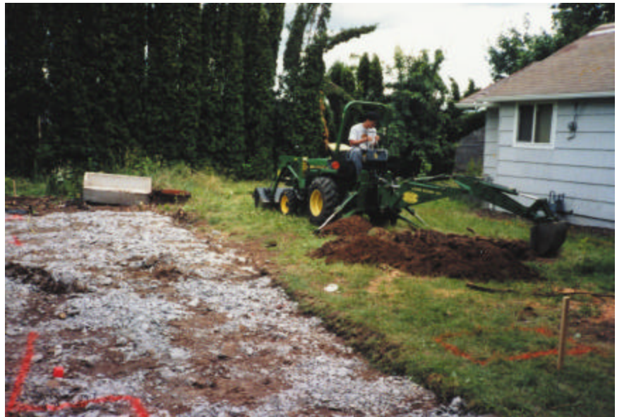
Wrestling with a tree stump while excavating for the new rental house
